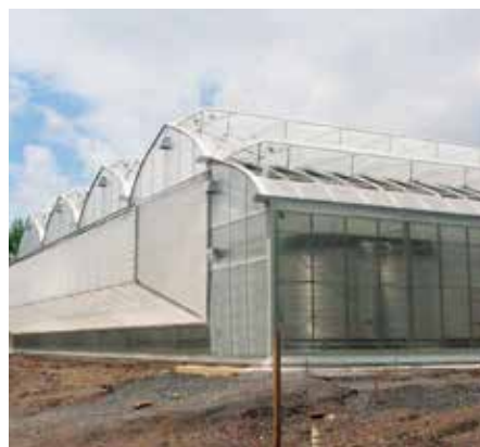
Mechanical ventilation (cooling pad)
